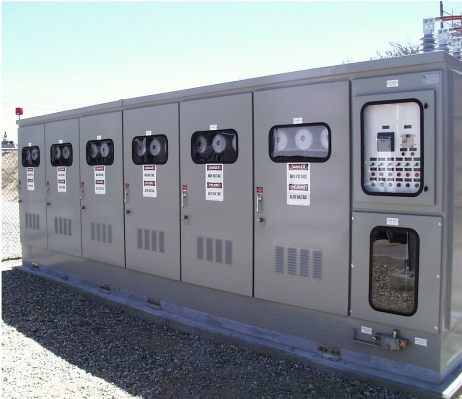
20 MVAR 12.47 KV 6 Stage Automatic Unit
