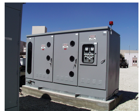
2.4 MVAR 2 Stage 15 KV Automatic Unit
