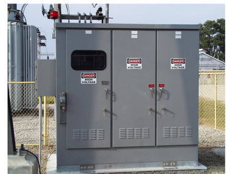
1.2 MVAR 5 KV Static Unit
