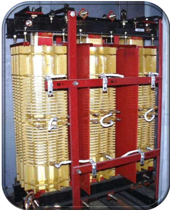
Three Phase 15 kV, Iron Core Reactor with Multiple Taps
