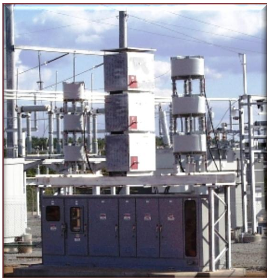
6.0 MVAR 5 th and 7 th "H" Type Harmonic Filter for a 25,000 HP Gas Pipeline Compressor
