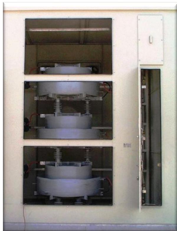
Single Phase 15 kV, Air Core Reactors with Multiple Taps
