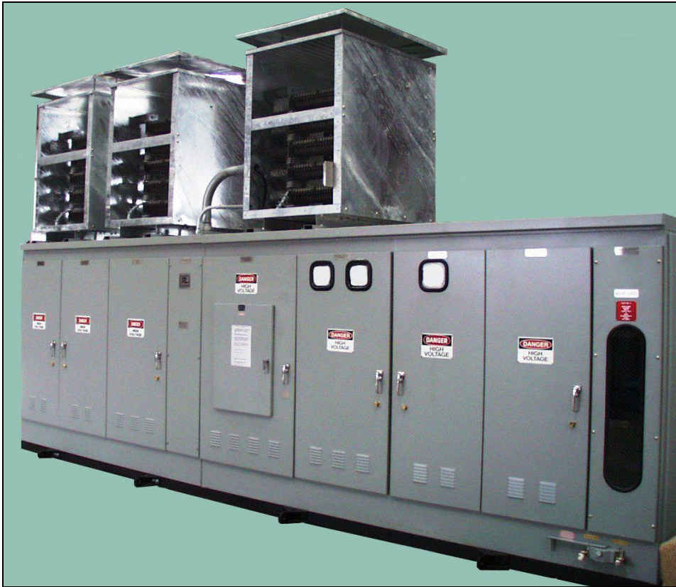
6.0 MVAR, 12.47 KV, Two Stage Automatic 5 th and 7 th High-Pass Harmonic Filter Assembly built for North Slope Alaska Operations
