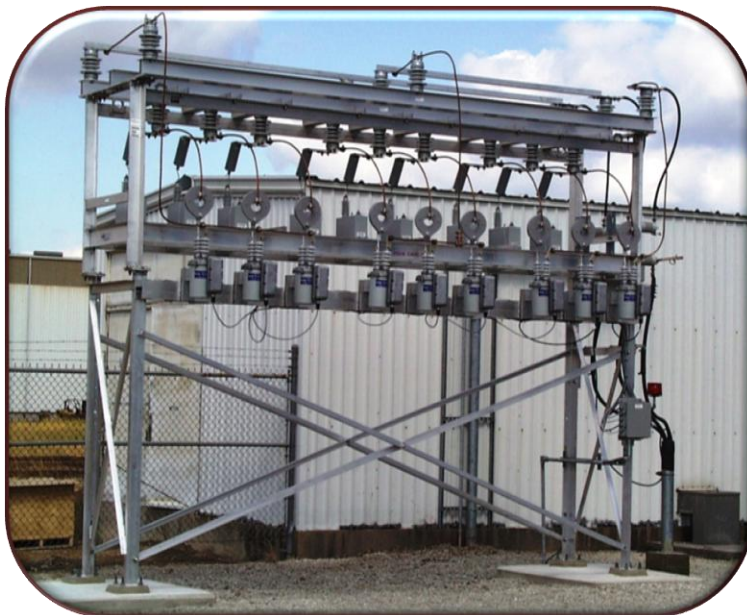
3.6 MVAR 12.47 kV, Three Stage Automataically Switched Substation Style Capacitor Bank.
