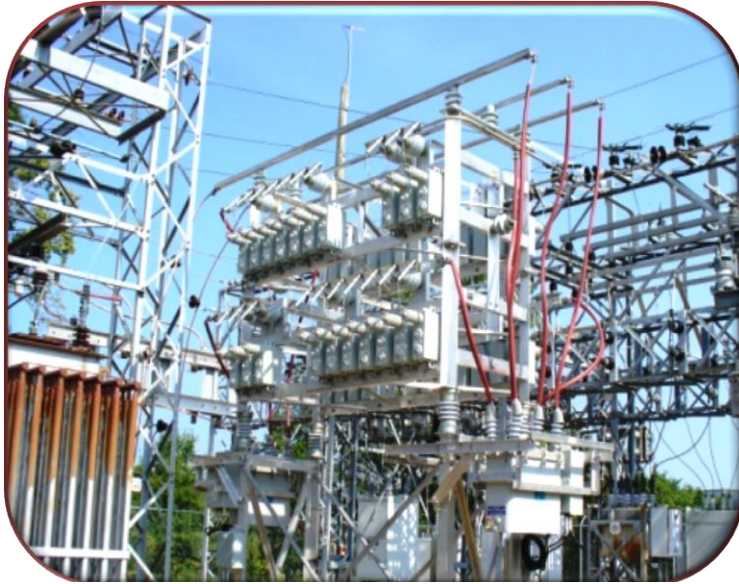
4.2 MVAR 4.16 kV, Two stage automatically switched substation style capacitor bank.
