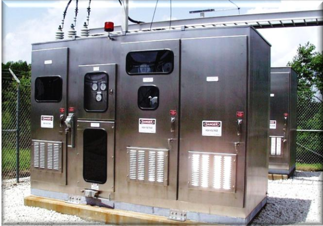
2.4 MVAR, 12.47 KV Power Factor Correction and Automatic 5 th Harmonic Filter Assembly in a 316 Stainless Steel Enclosure
