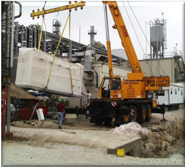
4.8 MVAR, 12.47 KV Automatic Power Factor Correction Capacitor Assembly
