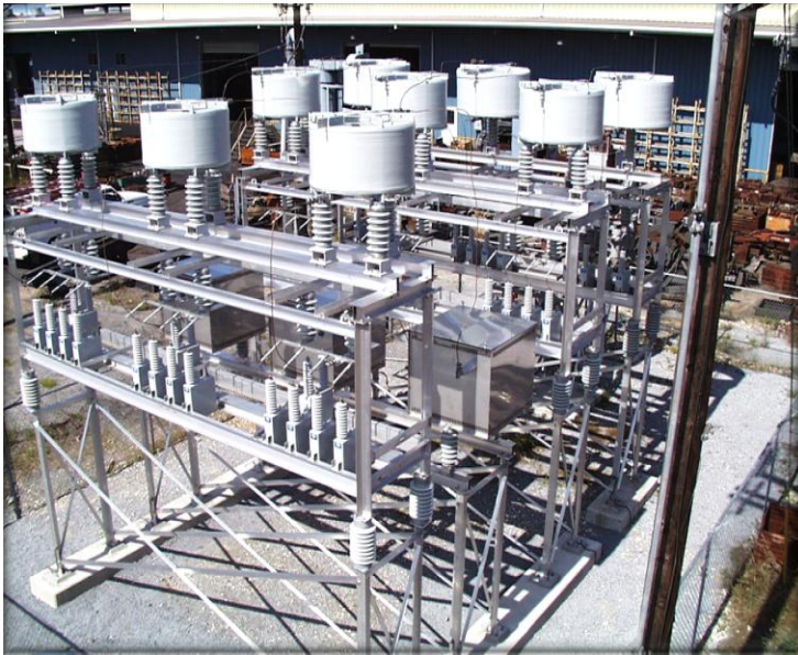
4.2 MVAR 34.5 KV, 5 th & 7 th Notch Filter and 11 th High Pass Filter with a "C" Filter
