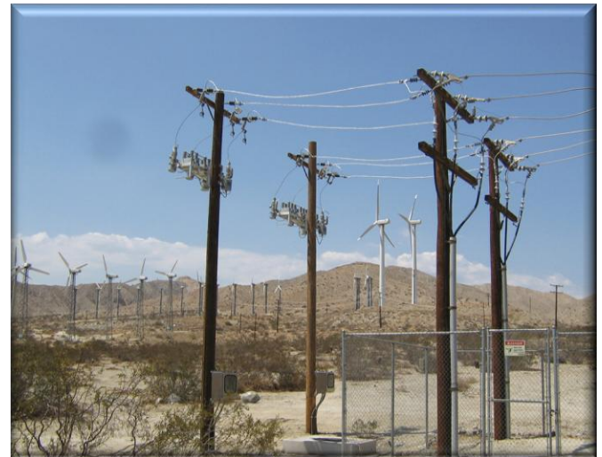
1.2 & 1.8 MVAR 12.47 KV Pole Mounted Units
