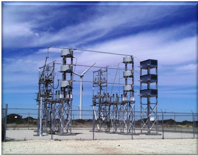
4.8 MVAR 34.5 KV Rated 5 th & 11 th High Pass Power Factor Correction & Harmonic Filter
