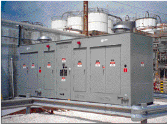
6.0 MVAR, 13.2 KV, TWO STAGE AUTOMATIC 5 TH HARMONIC FILTER SYSTEM
