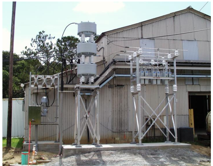
3.6 MVAR, 4.16 KV, ONE STAGE AUTOMATIC 5 TH HARMONIC FILTER SYSTEM
